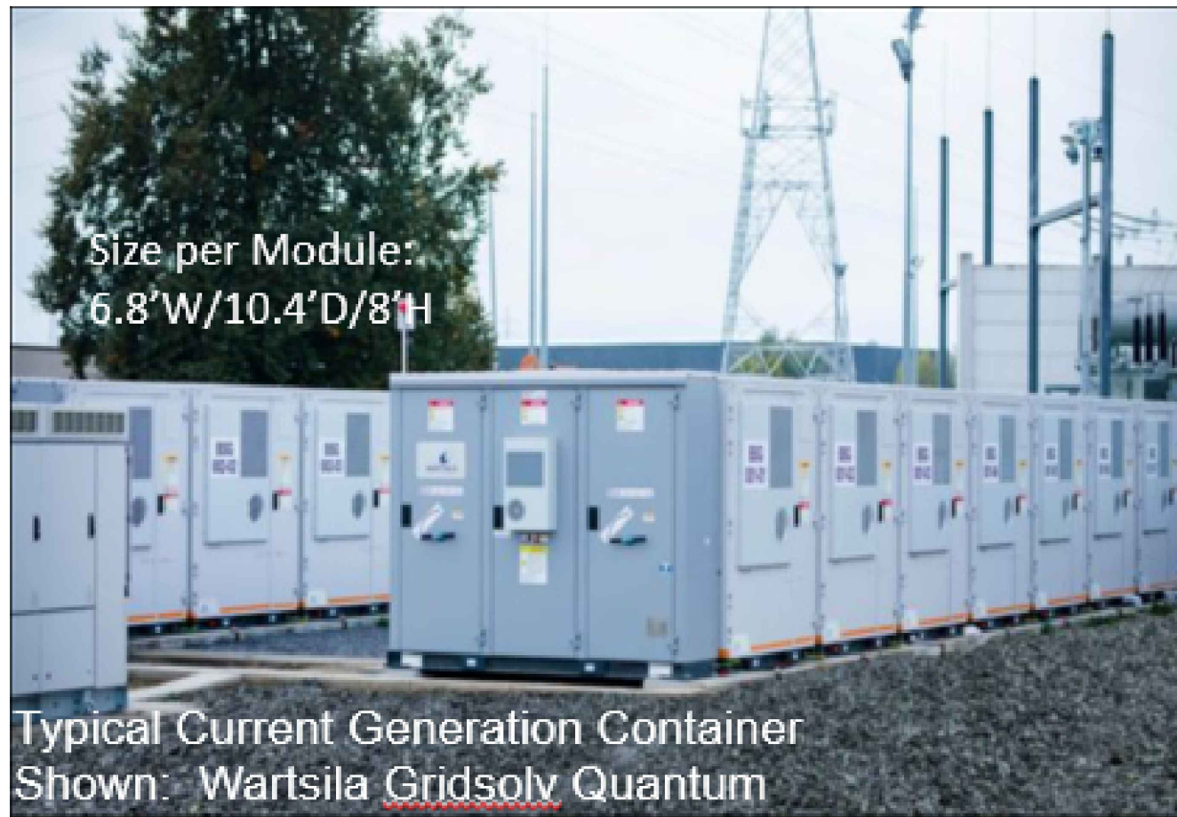
TYPICAL WARTSILA ENERGY STORAGE CONTAINERS
