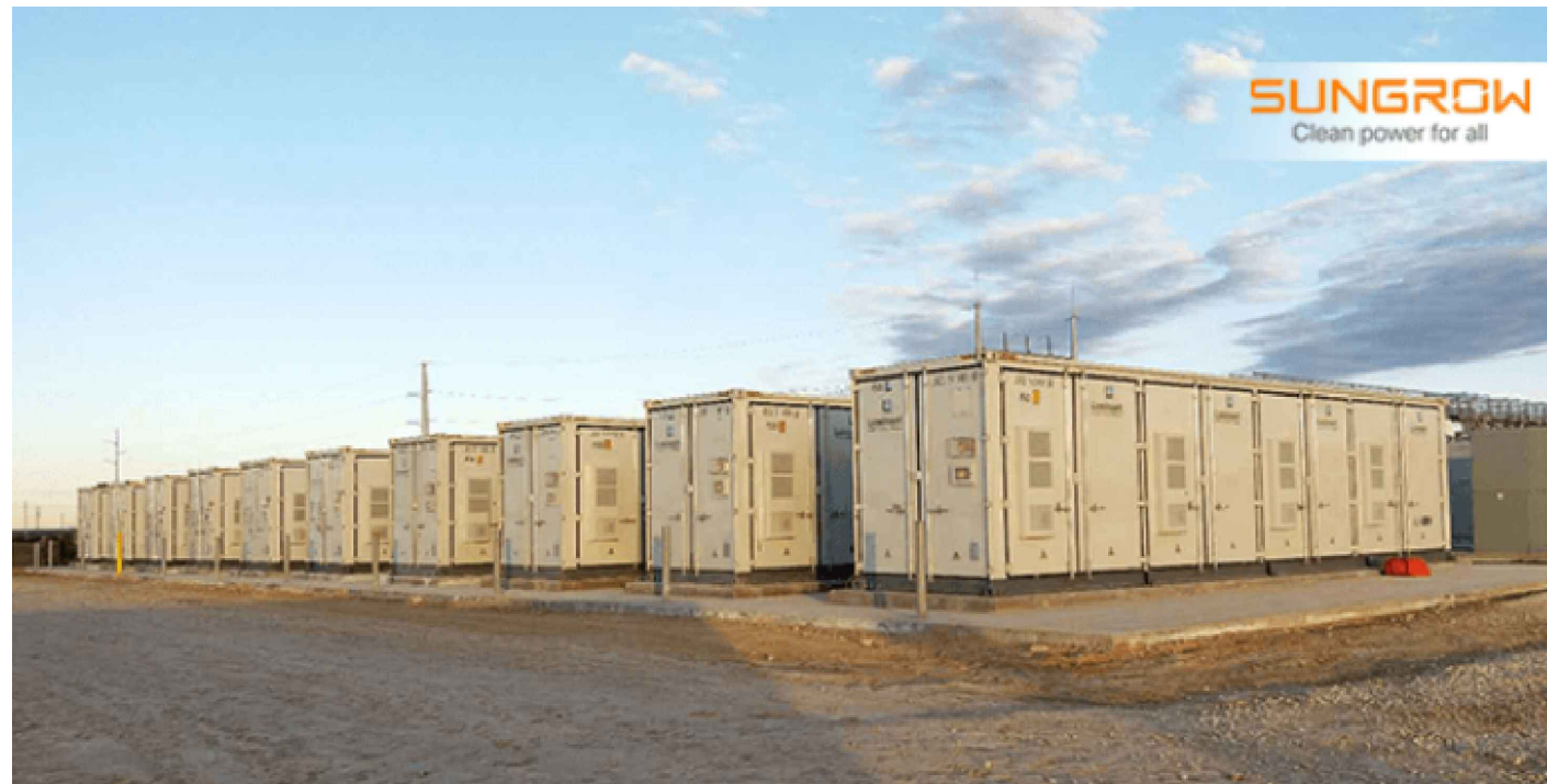
TYPICAL SUNGROW ENERGY STORAGE CONTAINERS
