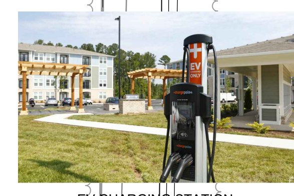
EV CHARGING STATION
